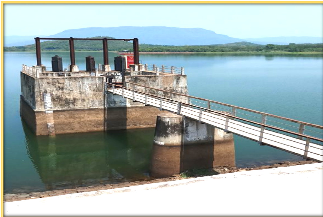
Head Regulator of Banapur Main Canal
