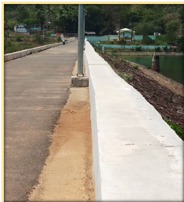
Repair of Upstream Slope Guard Wall at Salia Dam Under DRIP Project
